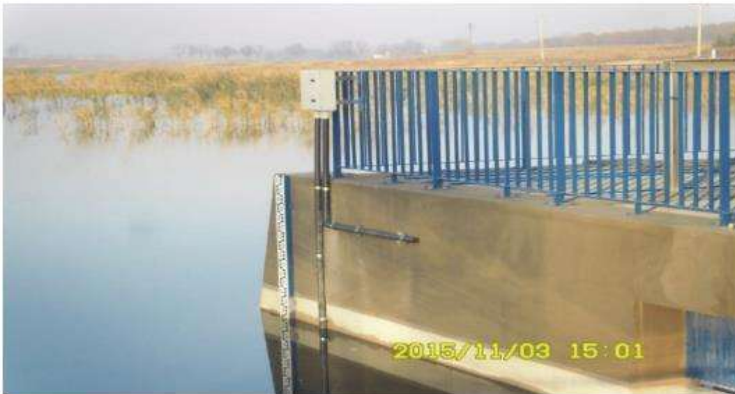
Fig. 2. A staff gauge with a hydrostatic probe installed at the damming structure at the outflow from the reservoir
